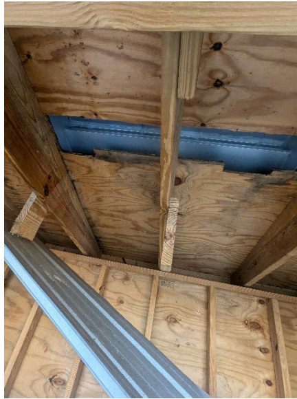
Photo No. 3 Post Test Underside
